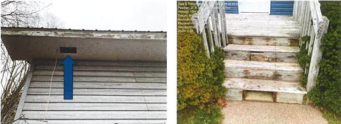
Figure 5. Left: Openings on the roof of the Alma Fire Department are susceptible to ember penetration. Right: Wooden steps with gaps and openings are located between two coniferous hedges, creating a potential vulnerability to fire spread.
