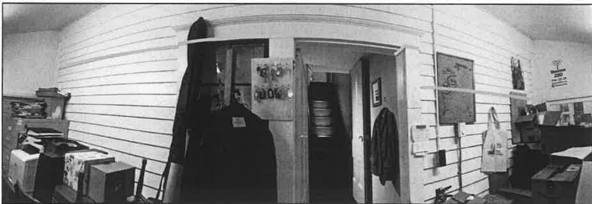
Figure 48: Inside wall of back porch, crack marked in orange
