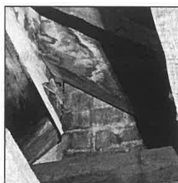
Figure 67: Moisture damage around leaning chimney stack in attic
