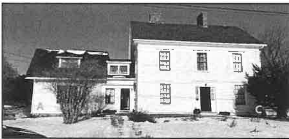
Figure 38: Gutter/drainpipe deficiencies at the south of the house
