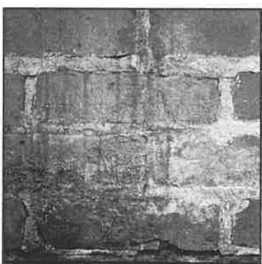
Figure 66: Moisture damage on second floor rear west bedroom fireplace
