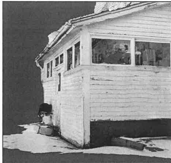
Figure 10: Ground slopes towards the building in many locations, generally matching areas with more deterioration
