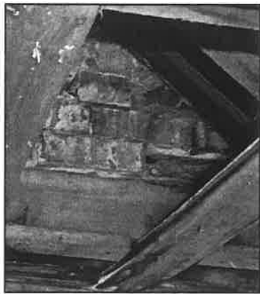
Figure 45: holes visible in west side of chimney, just under roofline
