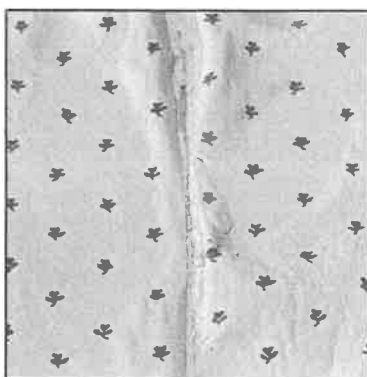
Figure 69: Moisture damage on second floor front east bedroom fireplace
