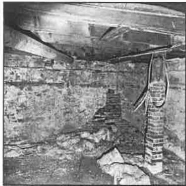
Figure 86: Interior of east cistern showing damage on south wall
