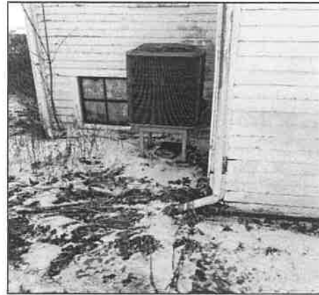
Figure 11: Wood siding too close to the ground and ground slope directing water to the building
