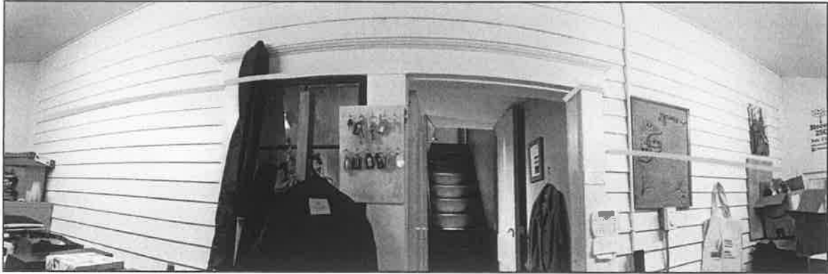
Figure 80: Highlighted crack along entire inside wall of porch
