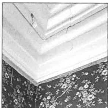
Figure 63: Moisture damage on ground floor dining room to the right of the fireplace
