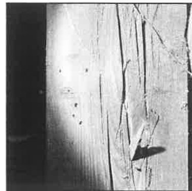
Figure 88: Damaged post in central area of basement
