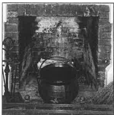
Figure 68: Moisture-driven deterioration in ground floor parlour fireplace
