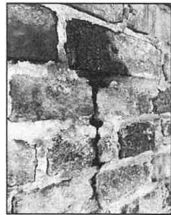
Figure 47: Detail of moisture deterioration on east side
