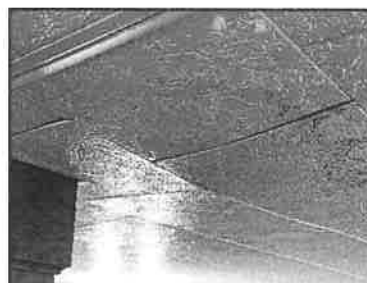
Figure 72: Major water damage and collapsing ceiling tile in apartment kitchen
