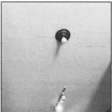
Figure 77: Cracking in ceiling of upstairs hall
