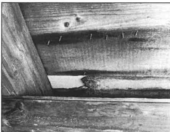
Figure 41: Blue roof membrane showing through deteriorated boards
