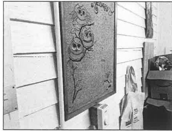
Figure 6: Horizontal cracking on inside porch wall
