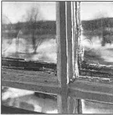
Figure 54: Typical mullion/muntin deterioration
