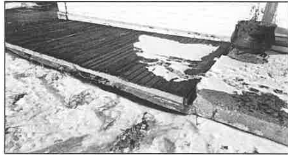
Figure 40: Deterioration visible on front step and decking
