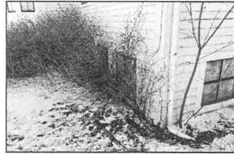
Figure 14: Plant growth abutting the house at one of the dampest regions in the basement
