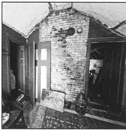
Figure 46: Extensive moisture damage visible on east side of chimney
