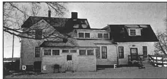
Figure 39: Gutter/drainpipe deficiencies at the north of the house
