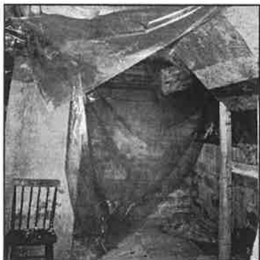
Figure 89: Failed vapour barrier and ineffective system
