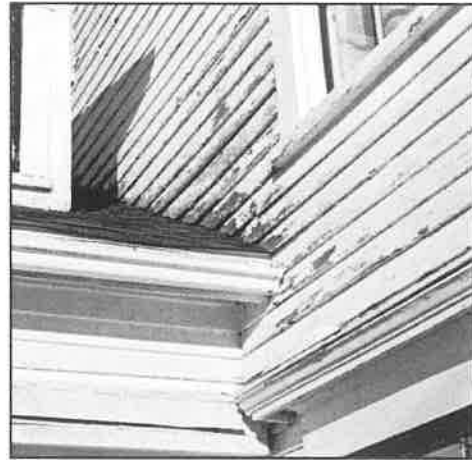
Figure 16: Example of paint deterioration
