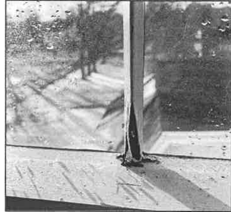
Figure 19: Condensation and deteriorated paint on west facing attic window
