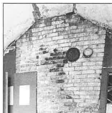
Figure 70: Moisture damage on central chimney stack in attic
