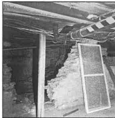
Figure 87: Broken wall of east cistern
