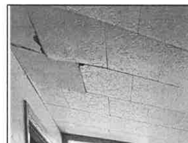
Figure 73: Major water damage and collapsing ceiling tile in apartment bedroom
