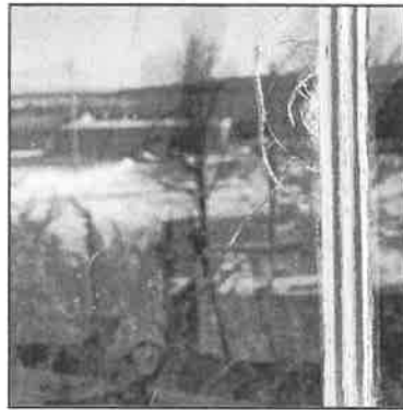
Figure 55: Broken pane, south window, front east bedroom
