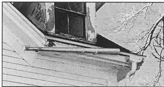
Figure 12: Failed guttering around east dormer
