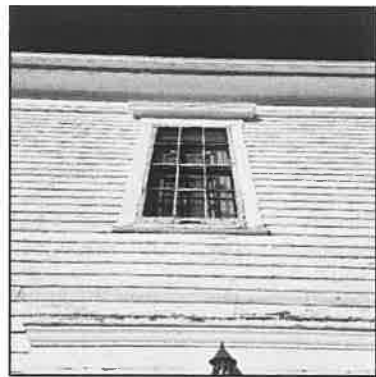
Figure 62: Exterior view of upstairs window and eaves, note that the window is not centered above the door lintel
