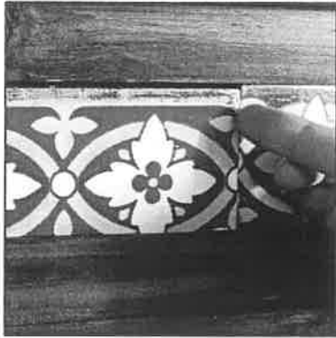
Figure 82: Loose fireplace tile
