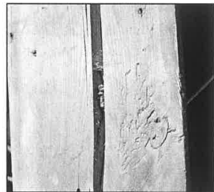
Figure 9: Check/Split in wood post. Some checking is normal in historic wood, but patterns and colour in depth suggests some areas are showing splitting failure
