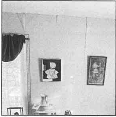
Figure 57: Peeling wallpaper east wall, front east bedroom
