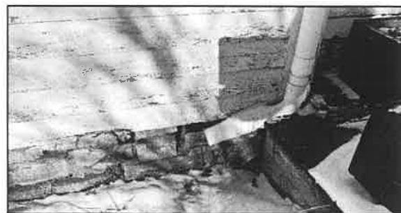
Figure 13: Downspout directing water directly onto foundation masonry
